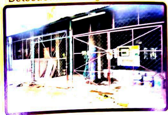
Lade & Generator Room
