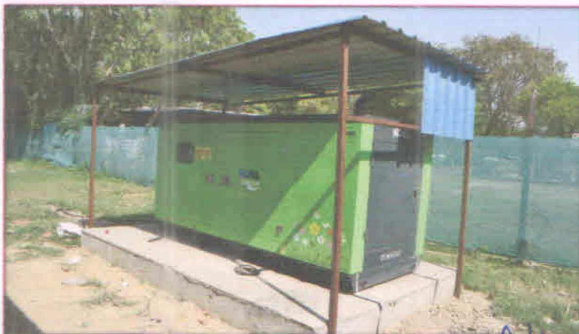
62.5 KVA GENR SET WITH OH SHED
